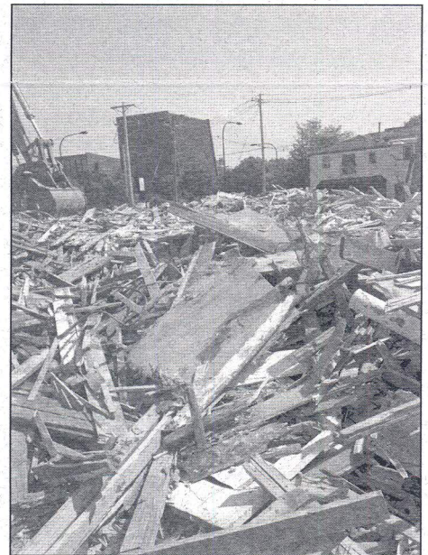
Demolition of 1203 West Oregon in August 2013; Krannert Center for the Performing Arts and Espresso Royale in background
