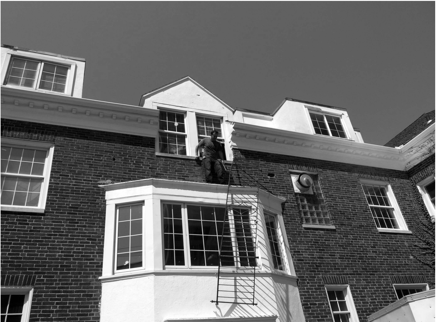
Daredevil Dan Leasure single-handedly removes a cast-iron railing from the second floor of the TKE fraternity house.
