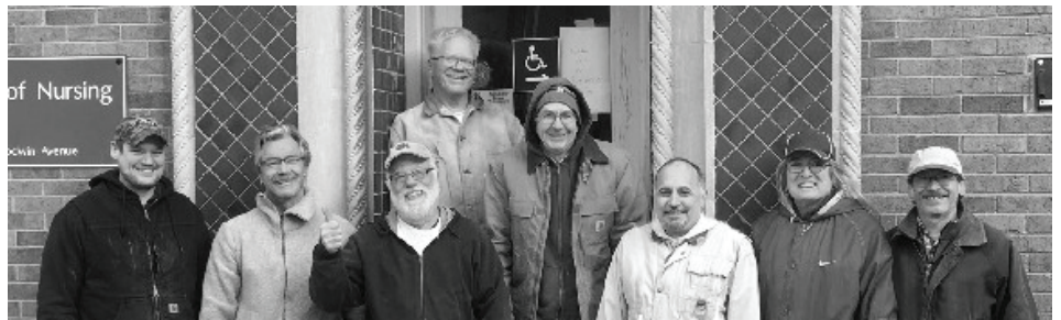
Salvage crew at 408 South Godwin Urbana, November 2016. We saved 50 doors as well as the two cast iron balconies.
