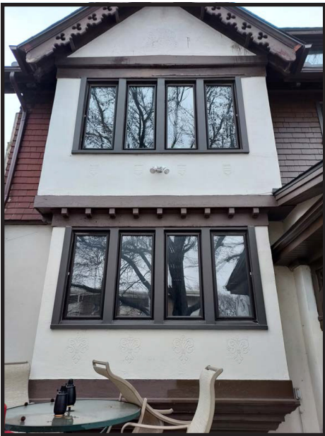
Detail, east gable, north elevation. Decorative bargeboard and dentils are visible. Façade/north elevation.
